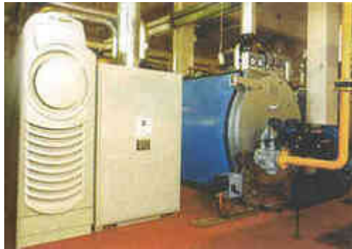
FIGURE 8: Capstone Microturbine - Generator System
