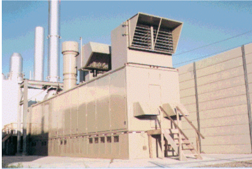
FIGURE 2: Steam Powered District Heating Cogeneration Plant
