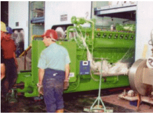
Reciprocating Cogeneration Engine (Jenbacher)
