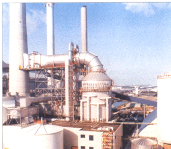
FGD plant with absorber and flue gas reheater
