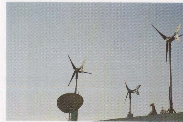
Wind Farm on Roof Top
