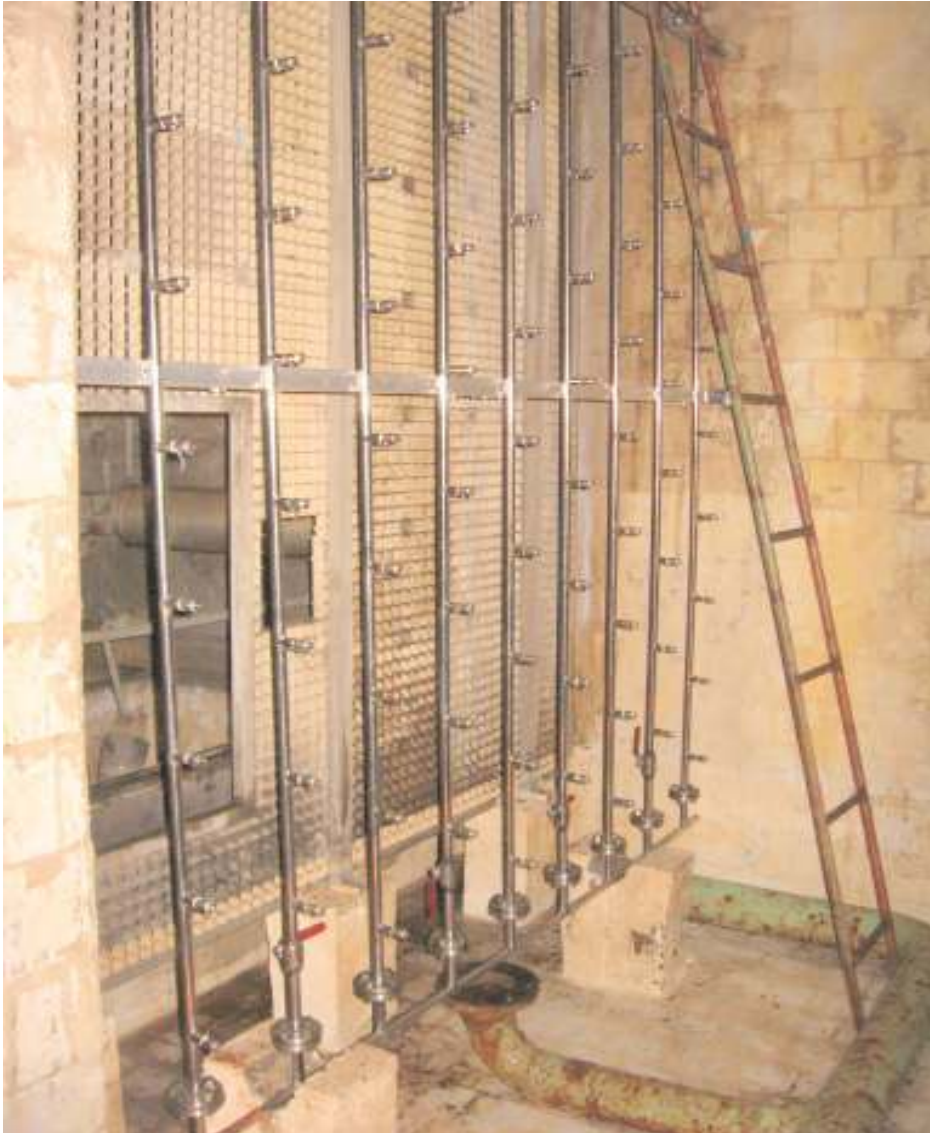
D. FOG BANK WITH SS PIPES & FOG NOZZLES
